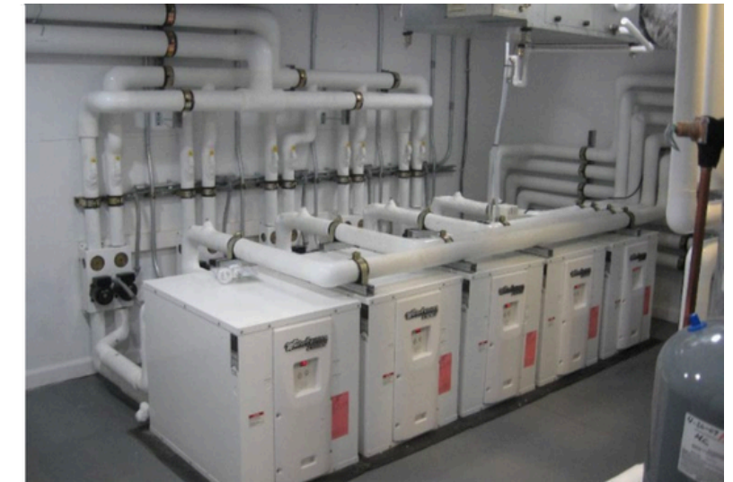
Ground-source heat pump system
